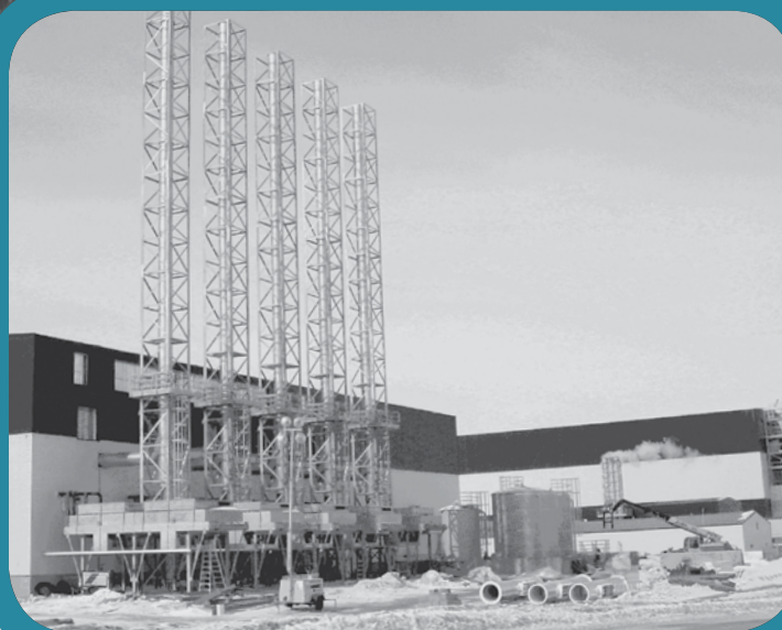
Generator & Fume Exhaust
