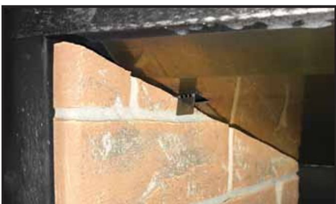
Figure 6 Left Refractory Handbend Tab
