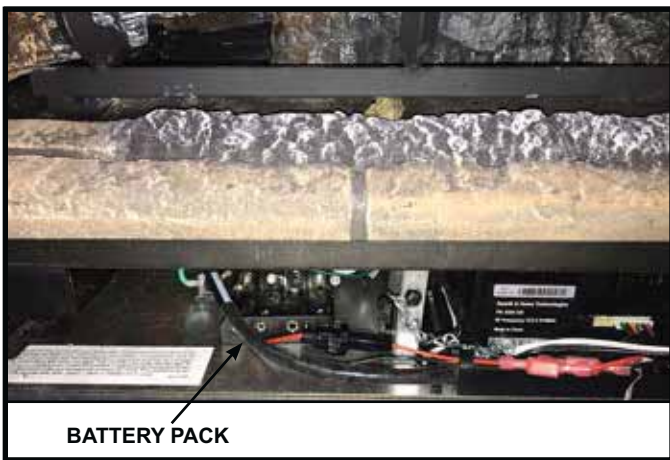
Figure 3.8 Battery Pack Installed
