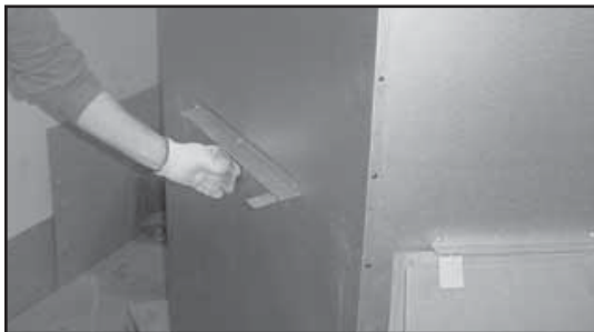
Figure 3.7 Bend Refractory Brackets Back Down
