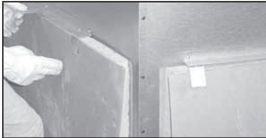
Figure 3.6 Unpacking Back Refractory
