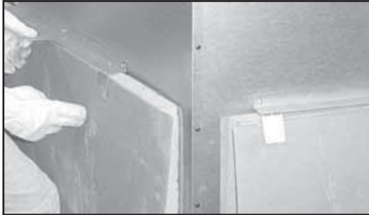
Figure 3.6 Unpack Back Refractory
